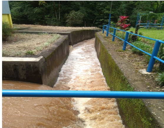
Gambar 2. Tailrace PLTMH Tombolo Energi
